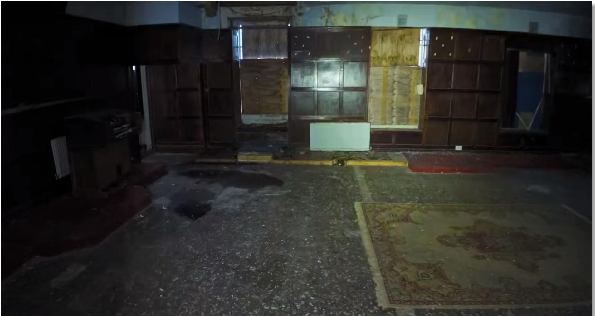
12. We are now looking at the top floor of the wing (above the Grand Salon). This would have been used for a Masonic room.
