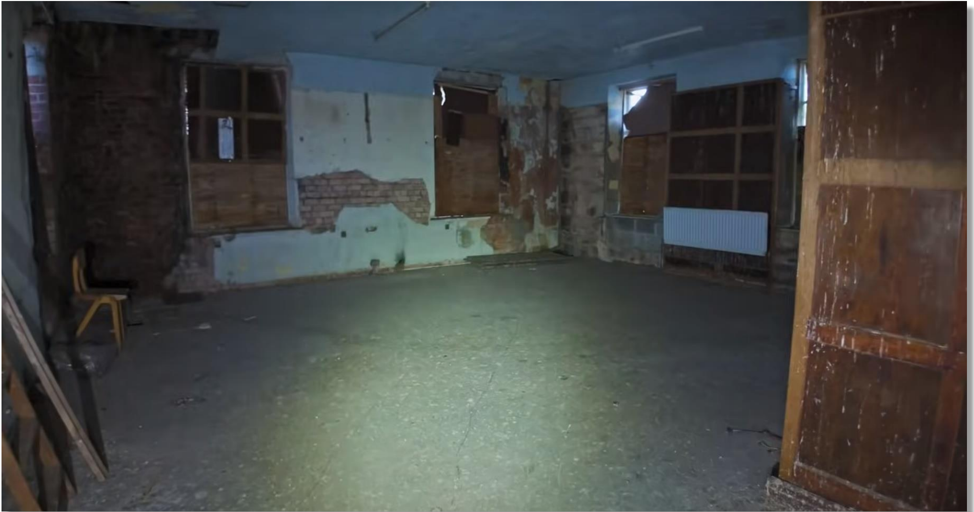
14. This is now the rear of the top floor side wing. It is in very poor state with missing window frames and water ingress.
