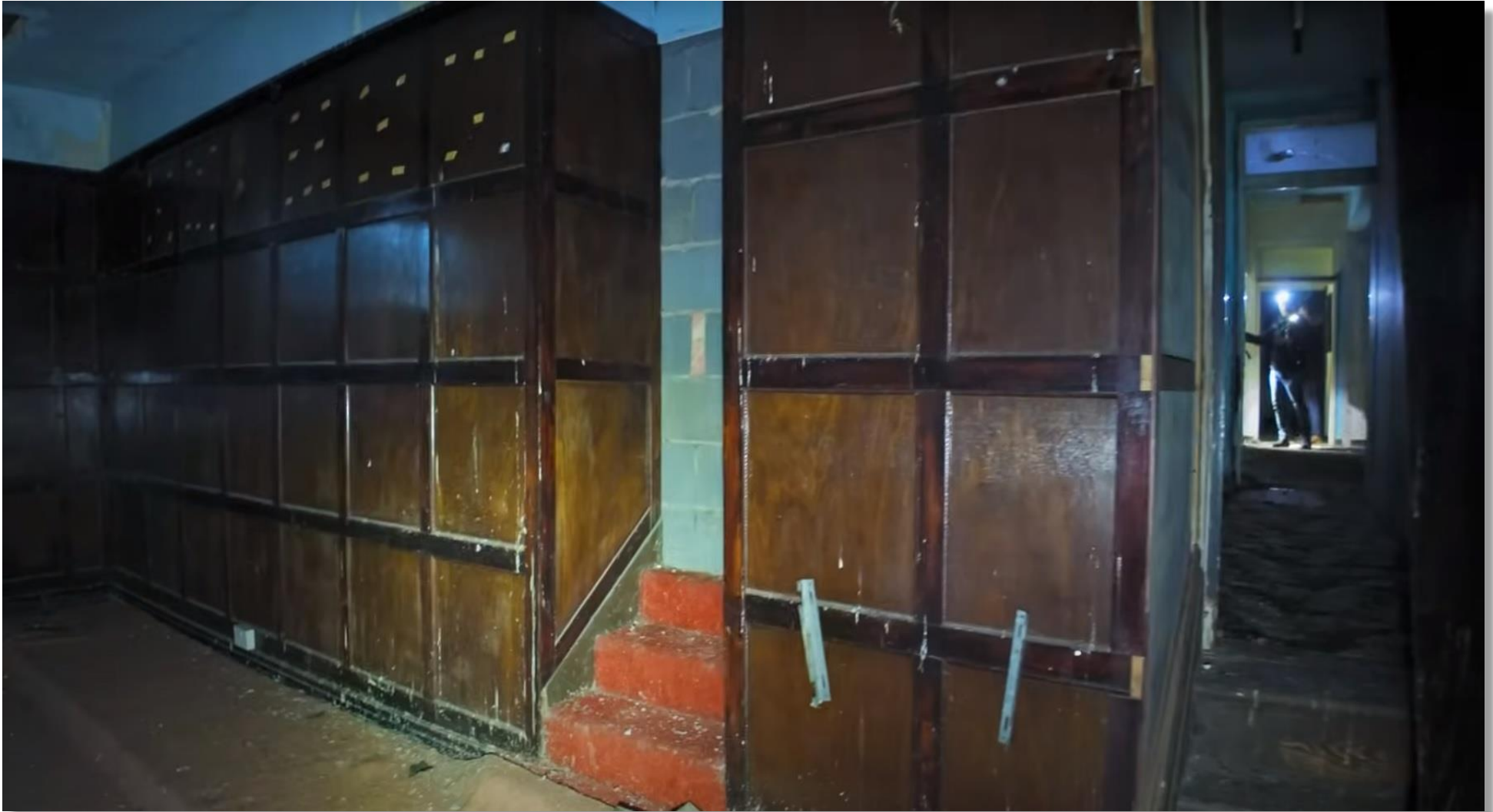
11. We are now in the side wing (top floor of the Great Salon) and viewing the blocked-up doorway on the left.
